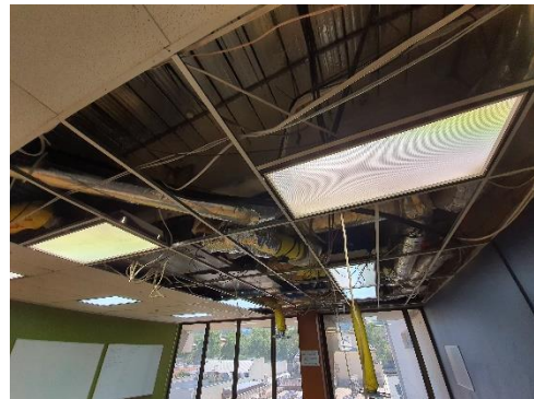
Image 4: 2 nd Floor affected area during interim clearance, prior to air conditioner repair.
